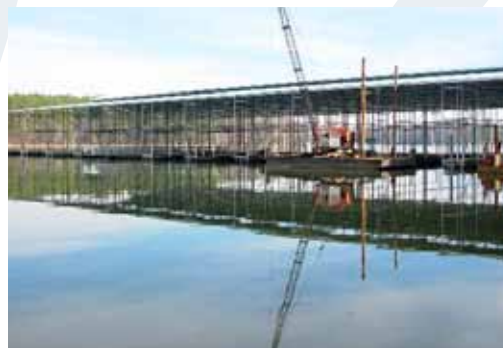
Here is a picture of Dock #700 under construction last year. Come see the finished product, it's amazing! I'd have a newer picture, but my camera is broken.
